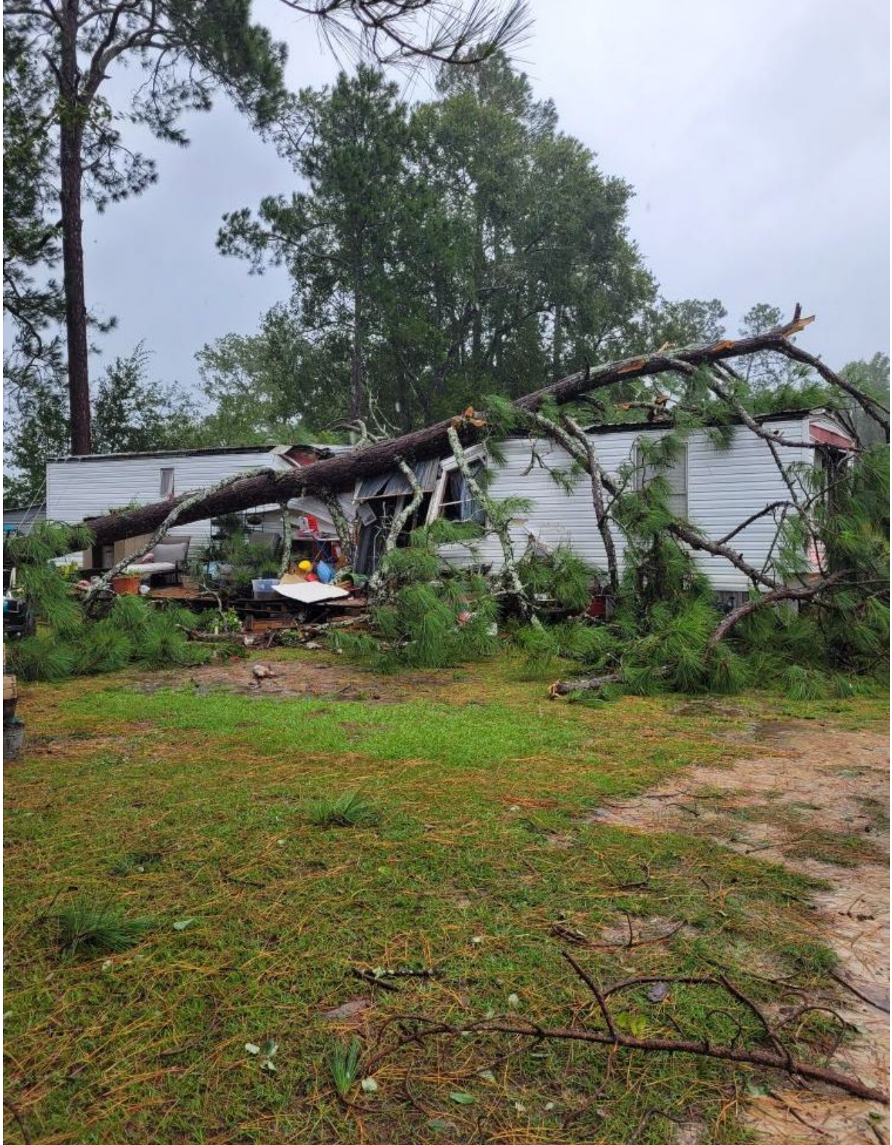
Hurricane Debby damage with tree on mobile home in Berrien County, Ga August 5, 2024
